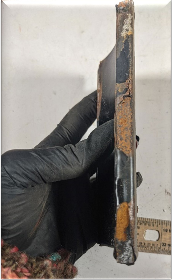
Disbondment of painted on coating
