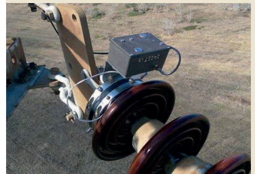
A suite of RF sensors have been developed for overhead transmission and substation applications. This is an example of a Clamp-on leakage current sensor installed on a porcelain disc insulator.
